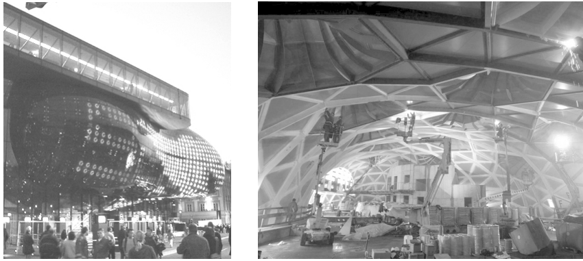
Fig. 2. Kunsthaus Graz. Left: the fluid body of the outer skin. Right: An interior view during construction, showing the triangulated and flat physical layers of the inner skin. Photo: Archive S. Brell-Cokcan.
