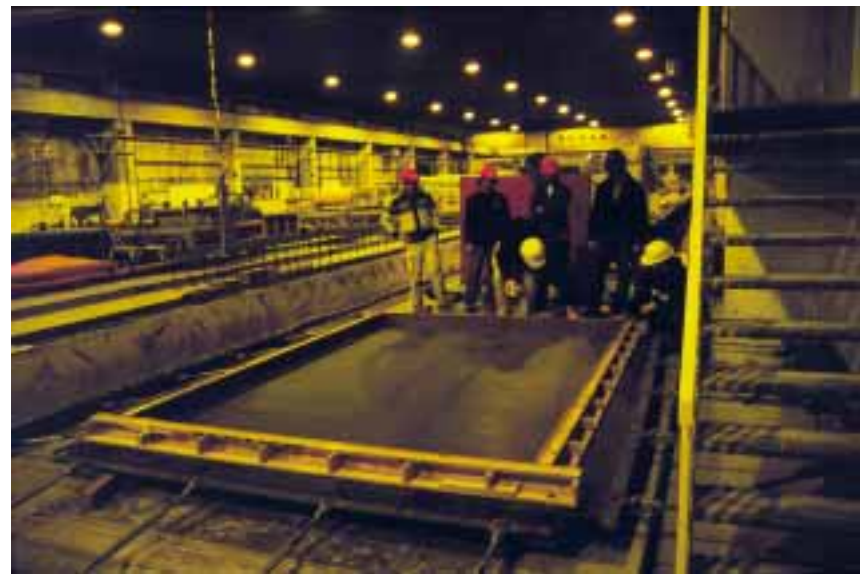
Figure 2. Complete formwork prior to placement of reinforcing steel: The fabric formwork membrane has been pre-tensioned over the lower frame and intermediate supports, and the upper frame is in place above the fabric membrane.
