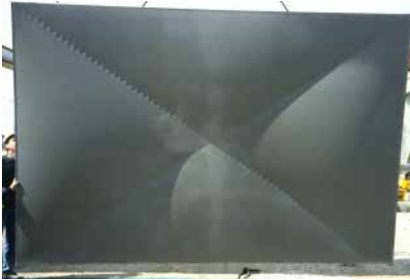
Figure 3. The 2.4 m X 3.7 m (8 ft. X 12 ft.) Concrete panel cast from the formwork illustrated in Figs. 1 and 2. Deflections in the formwork fabric have formed four funicular shell shapes in the unrestrained areas between the lower frame and intermediate X-shaped supports.
